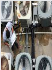
HVAC (DUCTING, CHILLED WATER, SPLIT UNITS)
